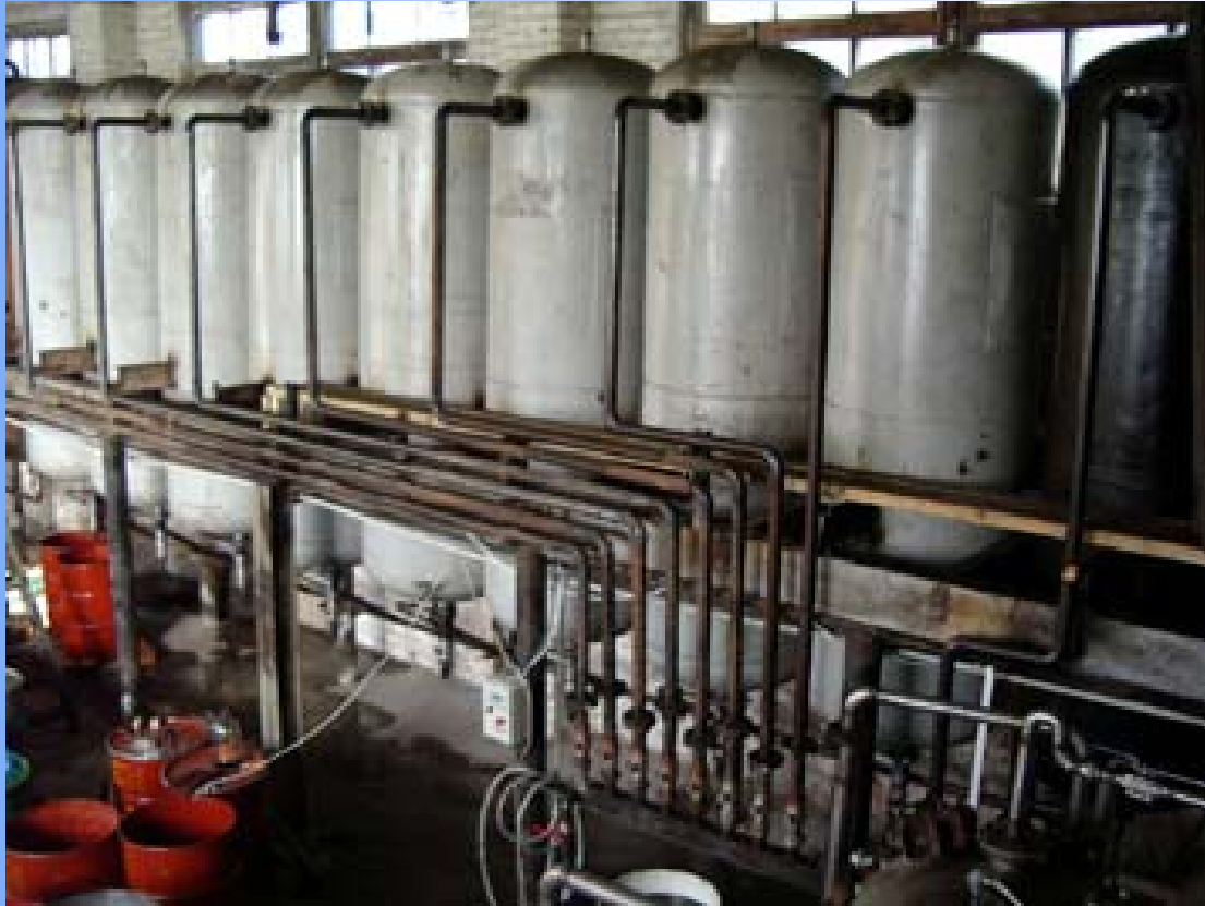
The installation in Jalgava, Latvia
