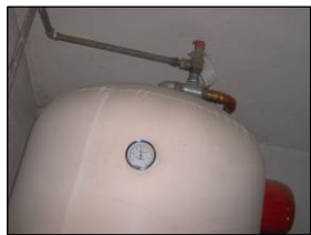
Tank san. Hot Water
