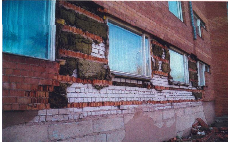
Photo 3 The results of lack of maintenance
