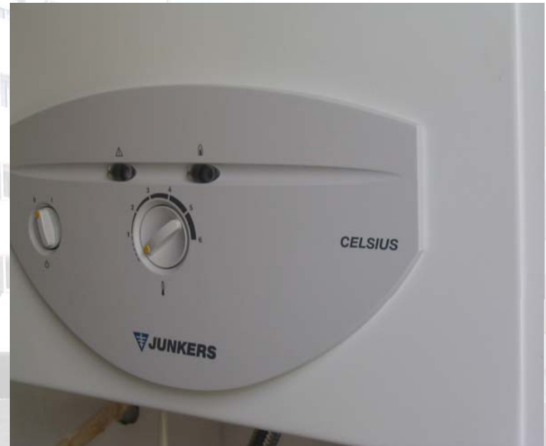
Gas hot water heaters for apartment top-up
