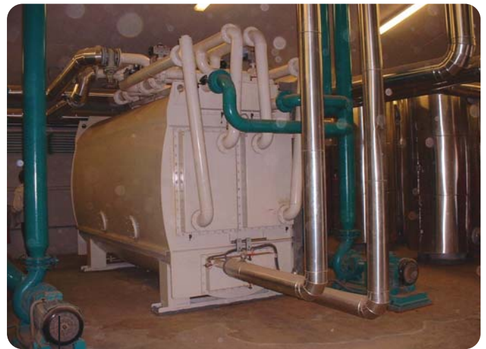
Figure 14 Adsorption chiller - Sarantis - Greece
