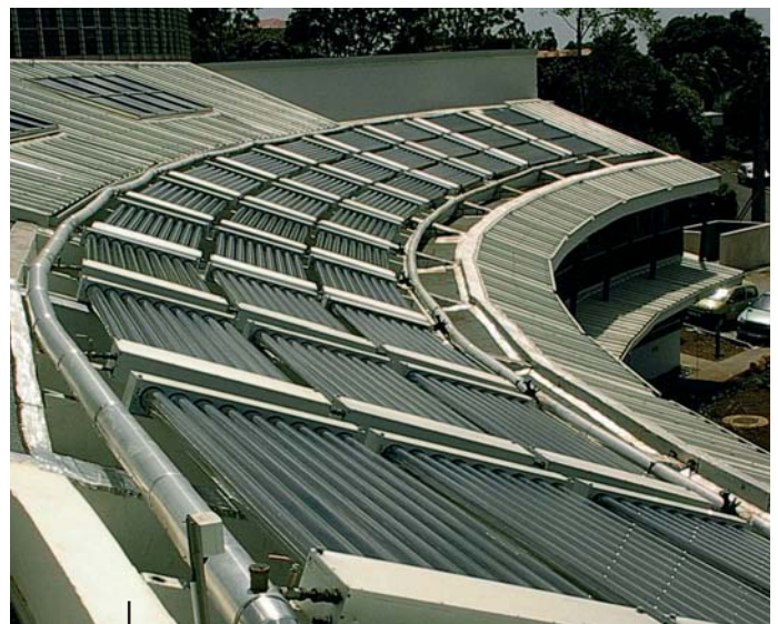
Figure 18 Integration of solar collectors on the roof of the DIREN (Guadeloupe, (F)).
