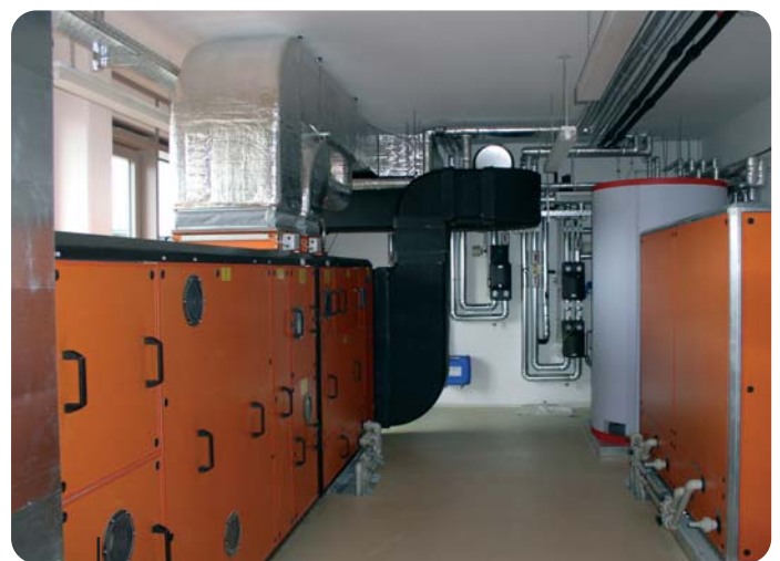
Figure 16 Liquid desiccant cooling system, installed at the new "Solar Building Innovation Center (SOBIC)" at Freiburg (D).
