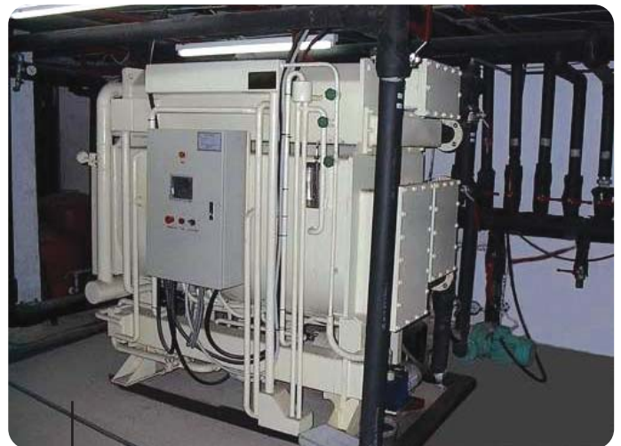
Figure 12 Absorption chiller – Rethimno village hotel - Crete
