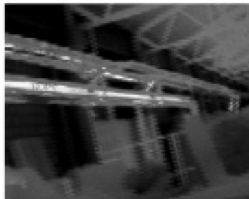
THERMOGRAPH 9: STEAM PIPES
