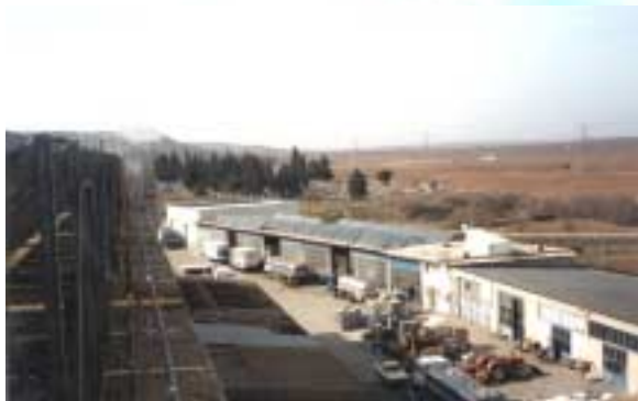
CPC + flat plate collectors on the roof
