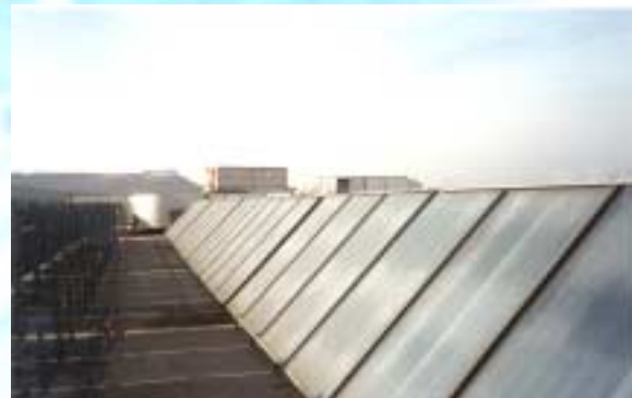
Selective flat plate collectors on roof
