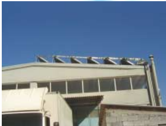
Solar collectors on the roof
