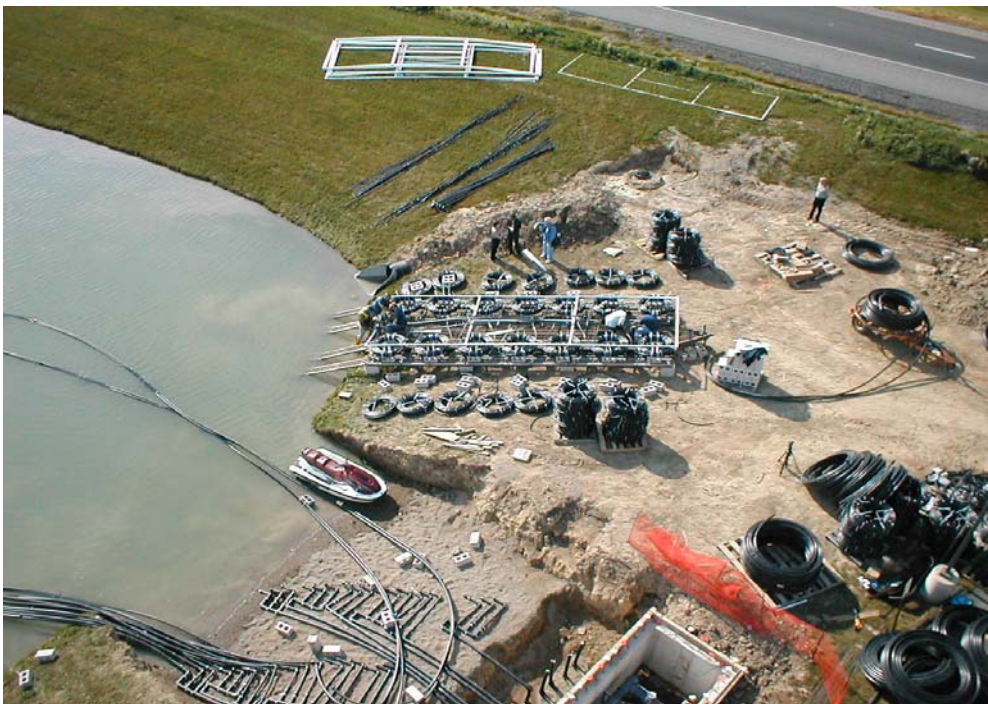
Fig. 1. Pond loop for system integration. Loop is high density polyethylene (HDPE), rated capacity is 150 kW, pipe bundles are fabricated from 19-mm pipe with spacers between loops. Each bundle has 92 meters of pipe. Header pipe sizes to and from building are 0.19 meters. Photograph courtesy of Geothermal Design Associates Inc. Ft. Wayne Indiana
