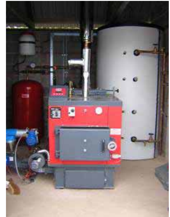
45kW pellet boiler
