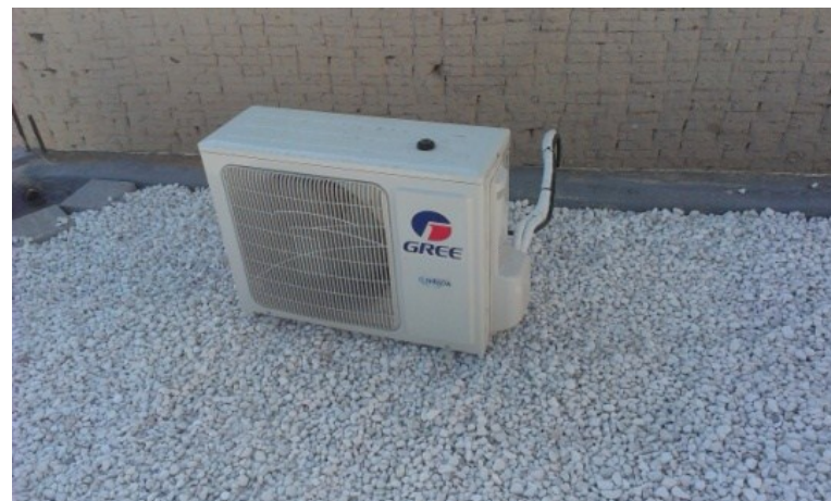
PP12 – New efficient air conditioning compressor
