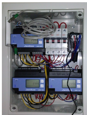
Smart metering devices
