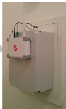
WiFi access point
