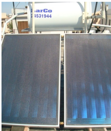
PP11 - New solar thermal water heater
