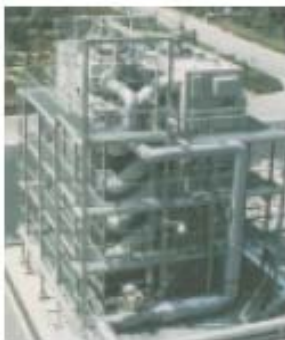
2,000 m 2 (0.5-mgd) vertically stacked MED plant in Japan Photo — Sasakura
