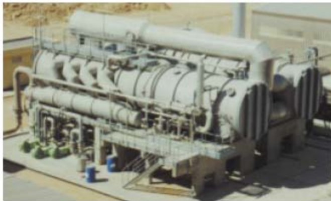
Thermal vapor compression unit in Saudi Arabia
