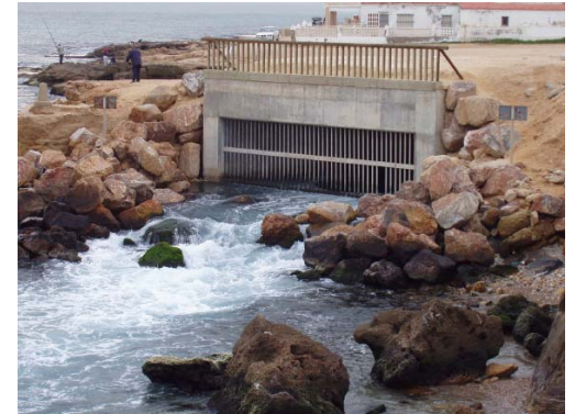
Brine outfall, Spain
