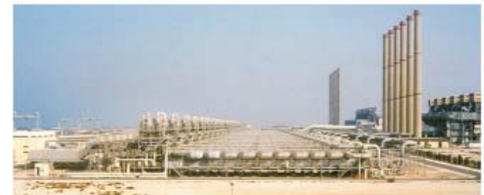
Dual purpose (power-water) facility in Saudi Arabia
