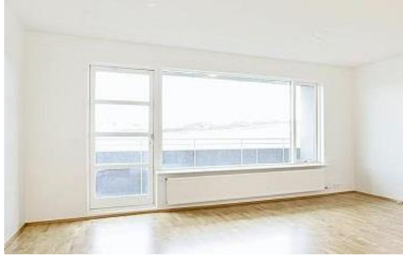
Typical radiator arrangement in an apartment
