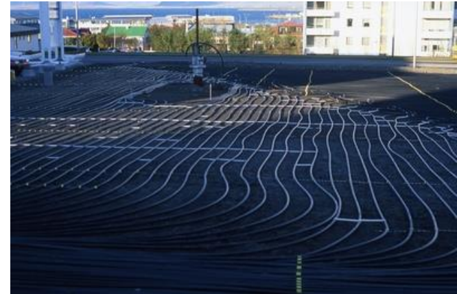
Snow melting systems are common in new parking lots ( http://www.nea.is/geothermal/direct-utilization/snow-melting/ )
