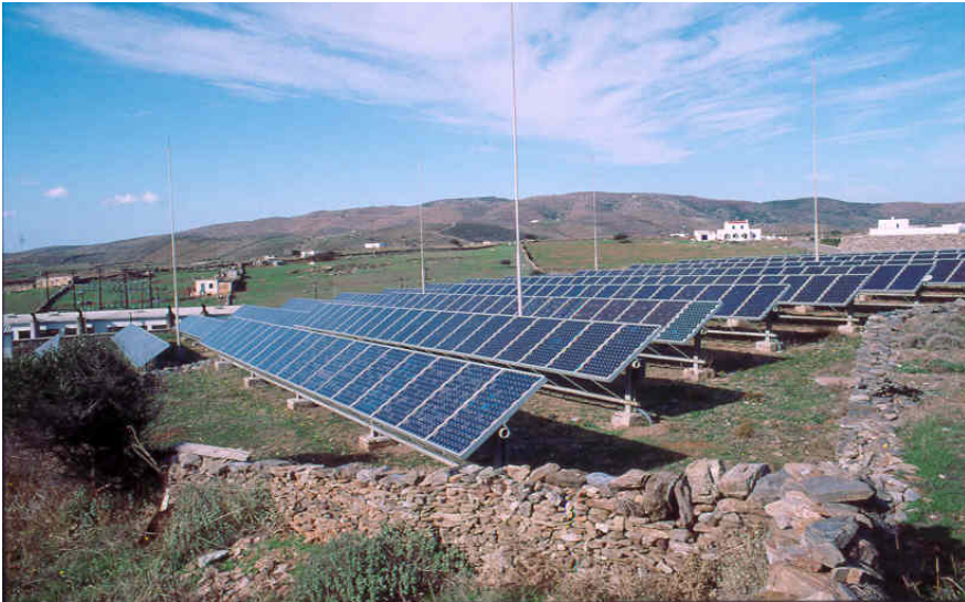
100kWp PV System at Kythnos island
