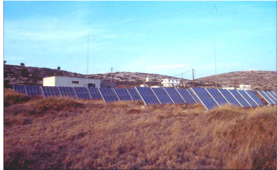
27.5kWp PV System at Arki island
