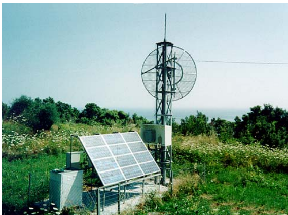
Figure 1: View of a solar-electrified telecommunication station
