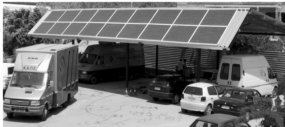
Figure 5: 5kW p grid-connected system, integrated into a parking shed.
