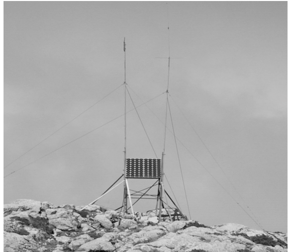
Figure 4: PV powered telecommunication antenna.
