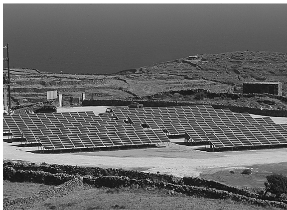
Figure 3: Central PV plant on the island of Sifnos, 60kW p installed power (THERMIE SE/0135/96 HE-I-D).
