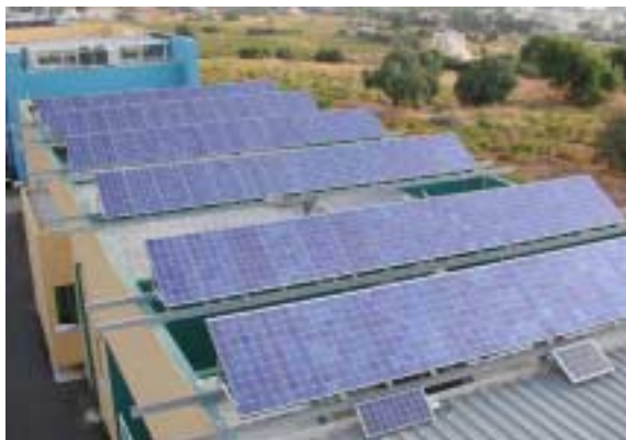
Fig. 5 CRES-4 PV system at the roof top of Building II
