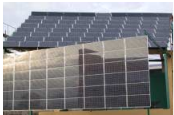
Fig. 6 CRES-5 and CRES-6 PV systems at Building II
