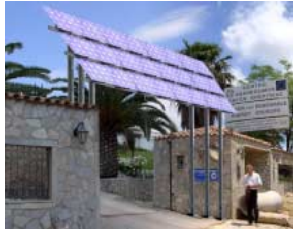
Fig. 2 CRES-1 PV system at the entrance
