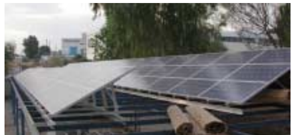
Fig. 3 CRES-2 PV system at the parking place
