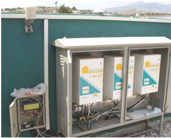
Figure 3: CRES-4 inverters, pyranometer and ambient temperature sensors
