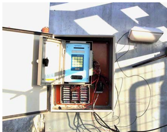
Figure 3. BMS set-up at CRES and data logger enclosure
