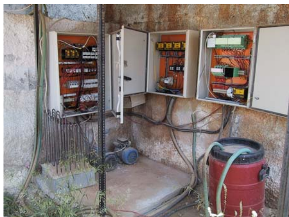
Figure 6: Distribution board of Interbus-S modules for the load simulator
