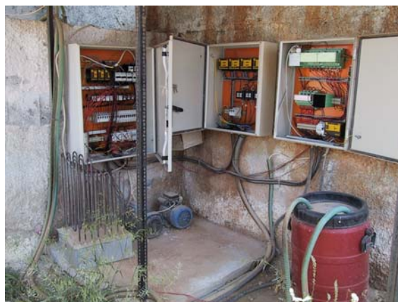
Figure 4: Distribution board of Interbus-S modules for the load simulator.
