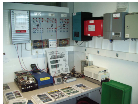
Figure 7: Install+RES training course laboratory with various inverters for on- and off-grid systems
