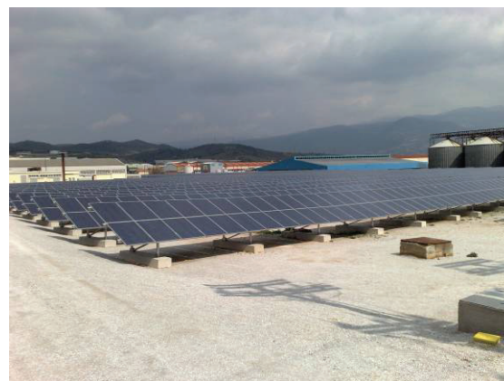
Figure 3: A 2 MWp PV system installed in the industrial zone of Volos.
