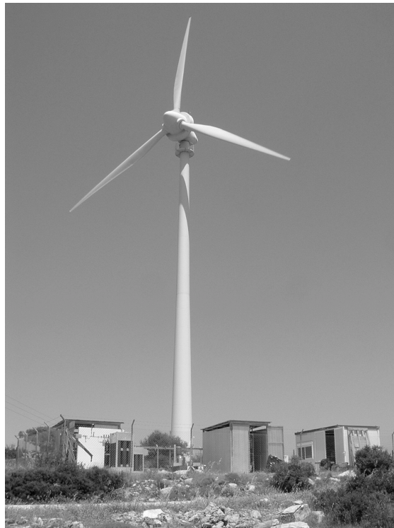
Fig. 2 Overall view of the wind – hydrogen installation
