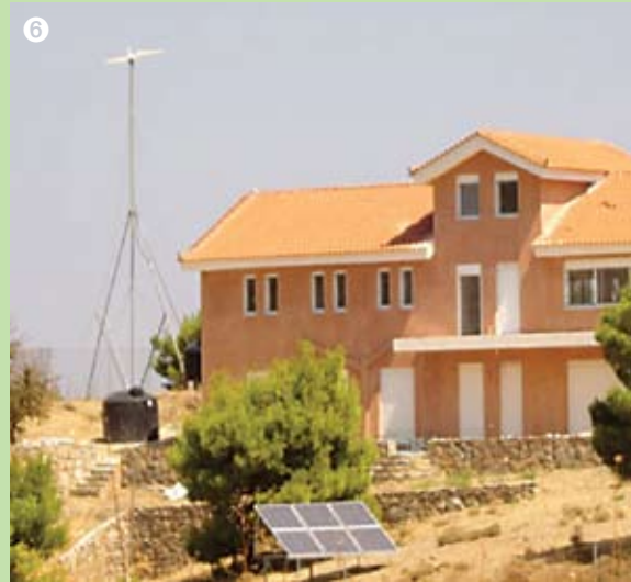
Hybrid system with 1,5 KW wind turbine in a house in Grammatiko, Greece Source: Alexakis Energy
