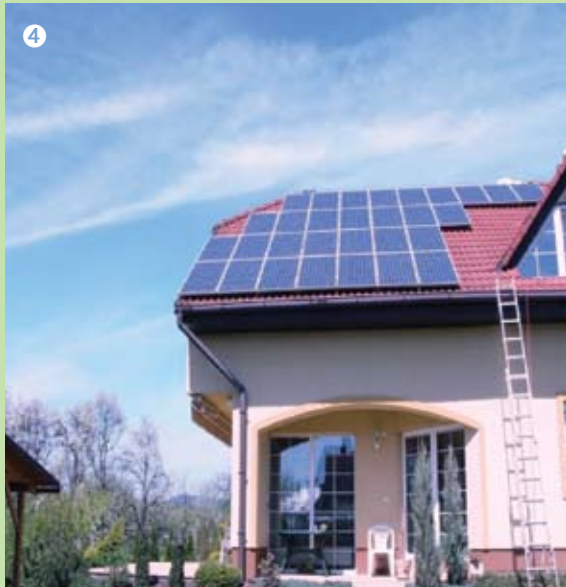
PV in house in Březová, The Czech Republic. Installed capacity of 4,35 kWp Source: Hitech Solar s.r.o.
