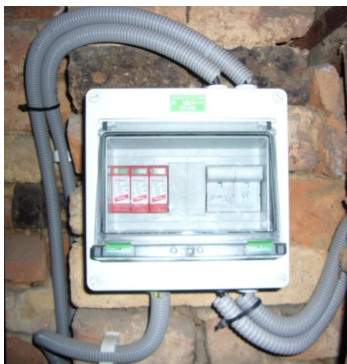
Transfer point PV to grid
