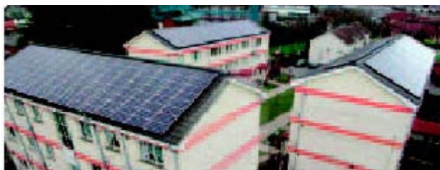
One of the largest PV projects in the UK
