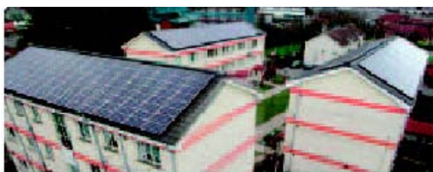
One of the largest PV projects in the UK
