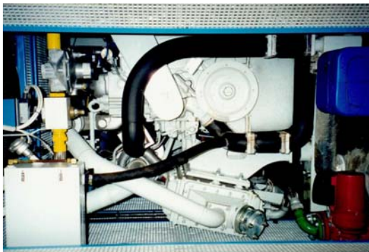
Cento 140 inside look – gas fired CHP
