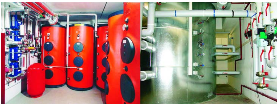
Figure 4.7 Tanks and piping for a multi-tank and a single tank system (source AEE)
