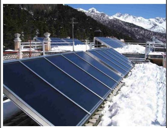
Figure 4.1: Solar plant in Pracatinat, Turin (Italy) (source: Ambiente Italia)
