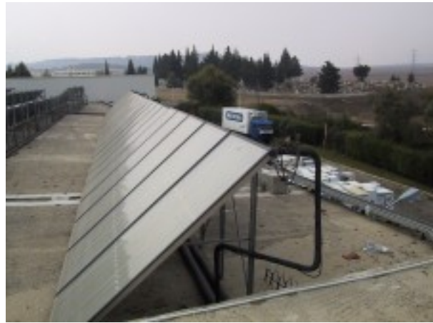
One collectors row in MEVGAL solar plant
