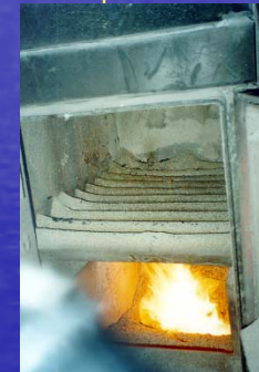
Hotel ATRION (2 olive kernel boilers 100.000 kcal/h & 120.000 kcal/h)
