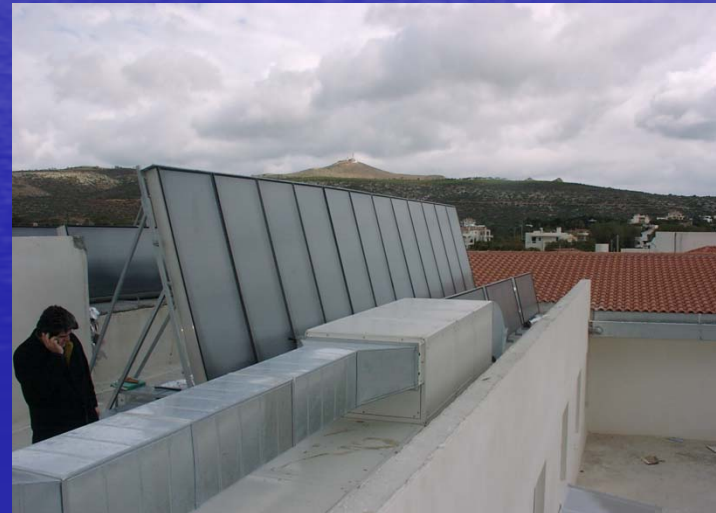
The solar air collector field for recirculation air heating (100 m 2 )
