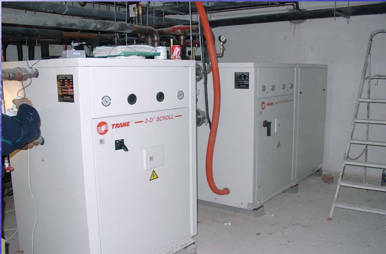
Two geothermal water to water the heat pumps (80kW και 130kW)
