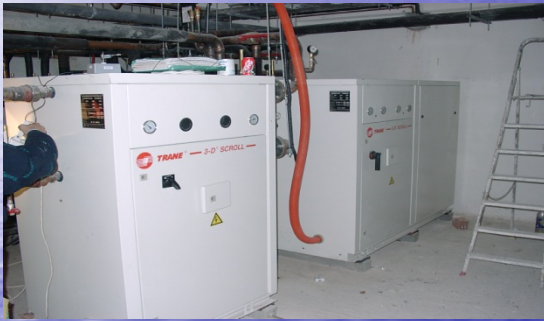
Hostel of the MEDUCA (Geothermal heat pumps with 24°C 1 x 120kW, 1 x 80 kW)
