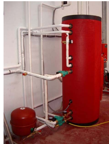
Storage tank, 500lt
