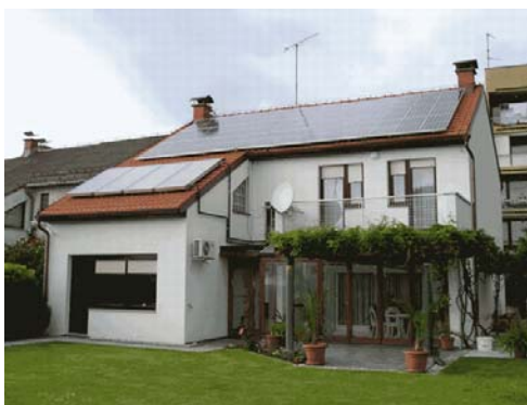
Figure 12 Solar roof in Špansko, Zagreb with flat plate collectors and photovoltaic modules (Source EIHP)
