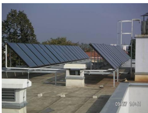
Figure 13 Flat plate collectors on roof of nursing home “Kuća Sv. Franje”, Odra, Zagreb
